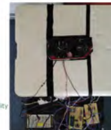
Fig.2: Picture of control room
